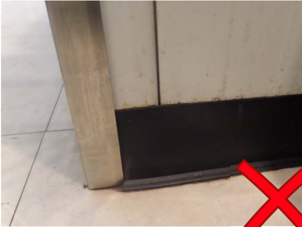
Non-compliant feather-edge skirting
