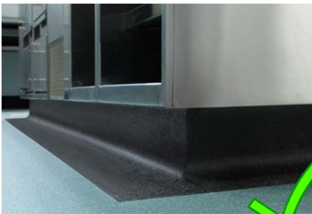
Plinth with seam-welded vinyl coving
