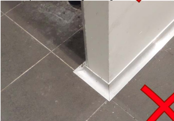
Non-compliant coving trim (non-rebated)
