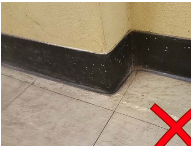
Non-compliant feather-edge skirting
