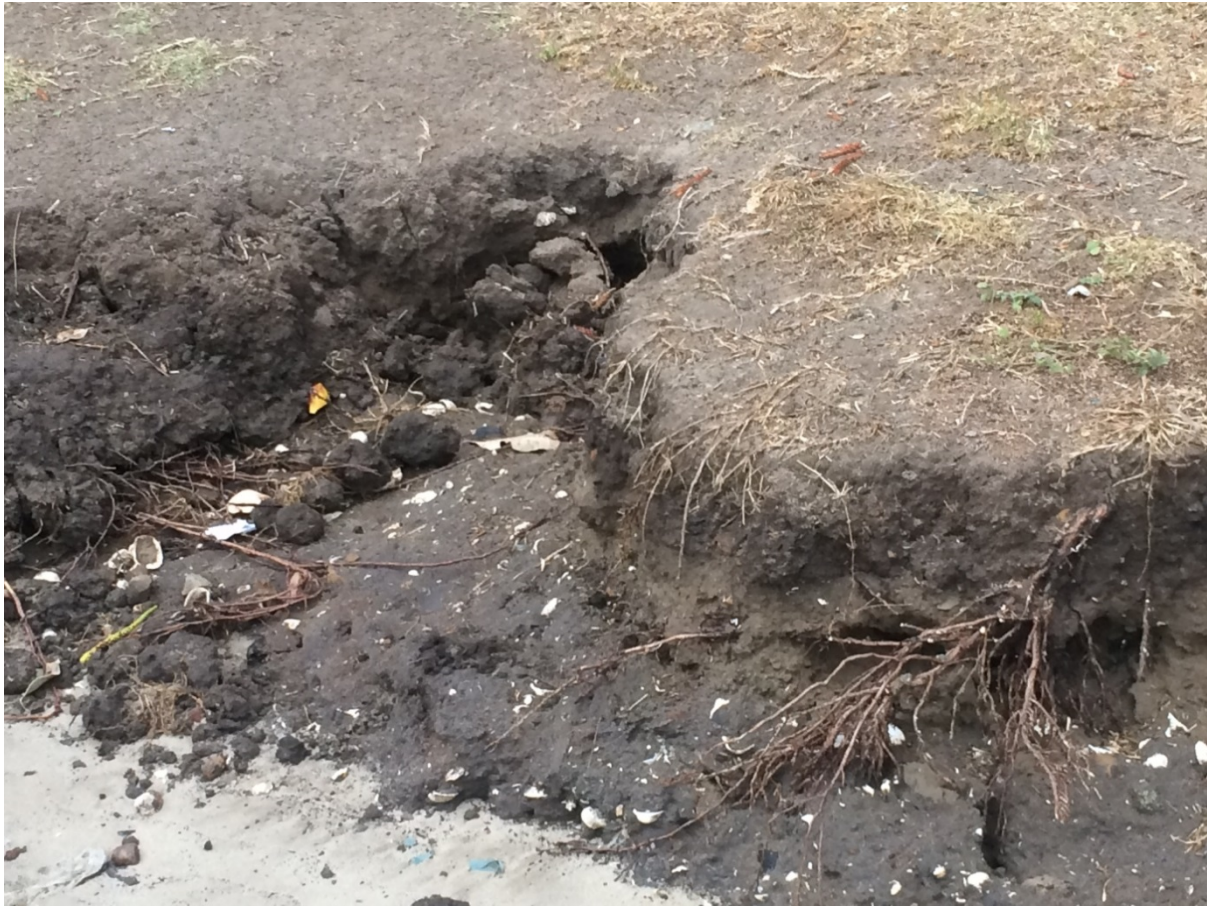
Figure 3: Example of foreshore erosion at Windang. Note that this portion of the foreshore is inundated at high tide. Photo taken 31 January 2017.
