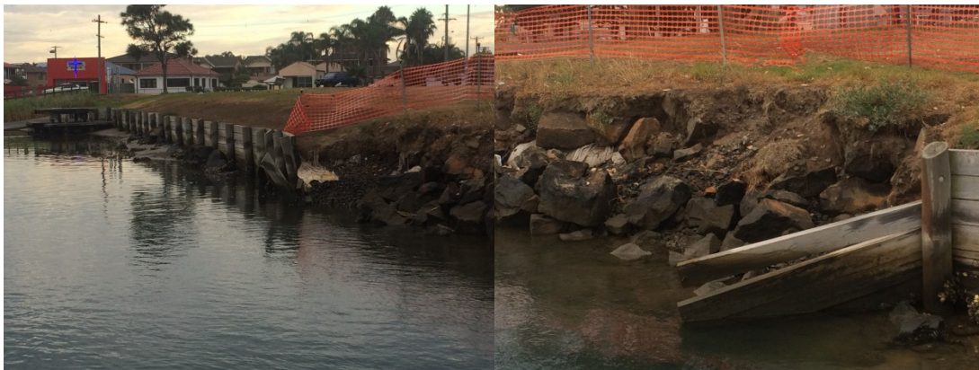
Figure 4: Failure of existing timber wall and subsequent erosion of bank due to loss of armouring at the Windang foreshore. Photo taken 31 January 2017.
