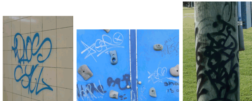
Examples of graffiti across a number of facilities at the skate park location. Some of the graffiti is offensive
