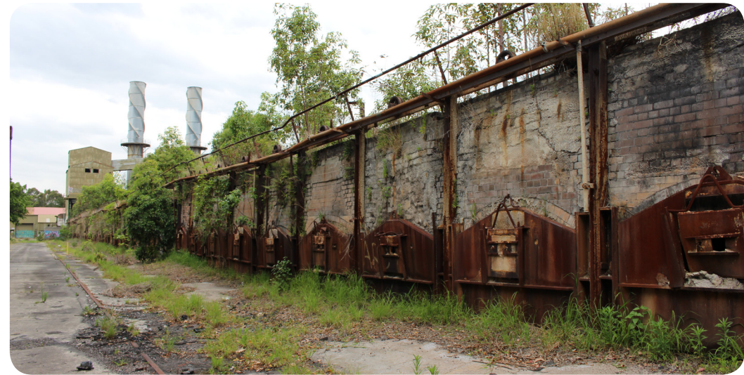
C1 COKE BATTERY
