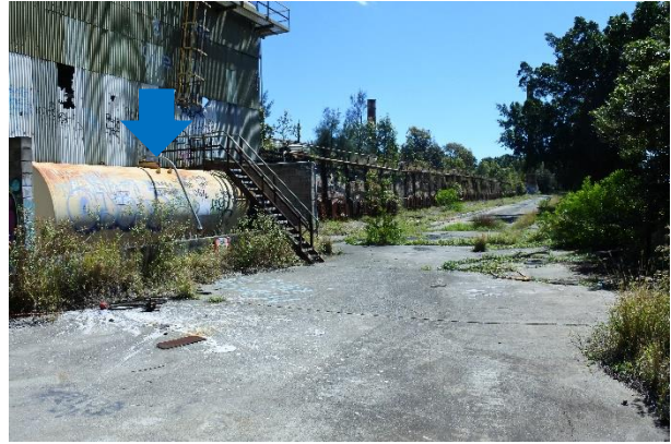
Figure 44 – Waste Oil Storage Tank
