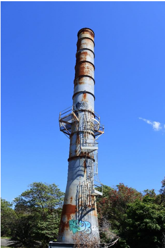
Figure 21 – Detail view of C2N stack.
