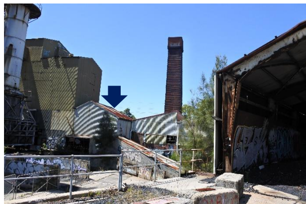
Figure 30 – View looking east showing grinding plant.
