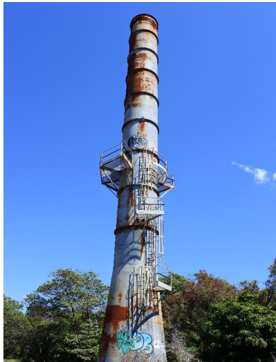
Figure 15 – Detail view of C2N stack.
