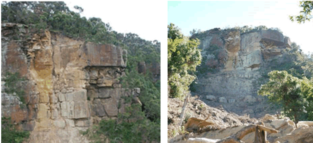
Rockfall below Five Islands Lookout showing overhanging area of the cliff. Source: Phil Flentje, University of Wollongong
