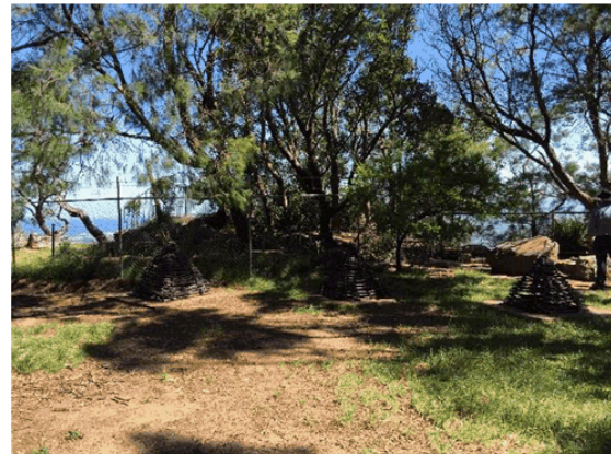
Access to Five Islands Lookout is fenced off due to cliff instability
