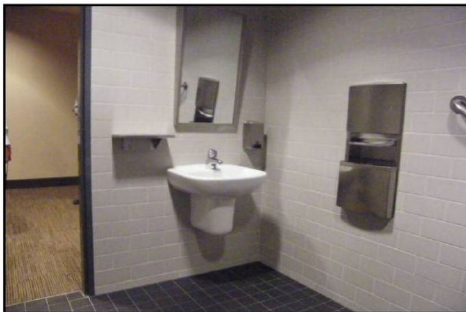
Figure 2729: The correct installation of a washbasin and other fittings, including a shelf as required by Table F2.4 of the BCA.
