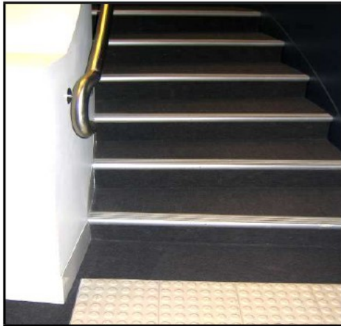
Figure 4113: Correct enclosed opaque risers with no overhangs which meet the requirements of stairways suitable for people with disabilities, under AS1428.1.
