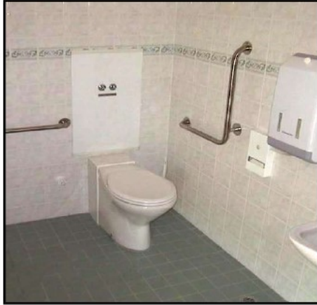
Figure 2830: The incorrect placement of the toilet paper holder too far forward of the WC pan, which forces patrons to lean excessively forward to get to the paper. This can result in patrons falling off the pan in attempting to reach the toilet holder.
