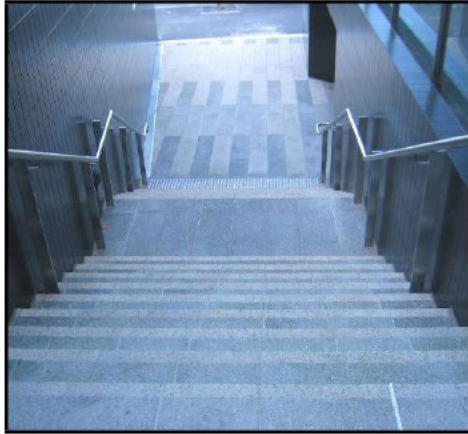
Figure 4618: The correct interpretation of the requirements for TGSIs on an intermediate landing with no handrail break: there are no TGSIs on the landing.
