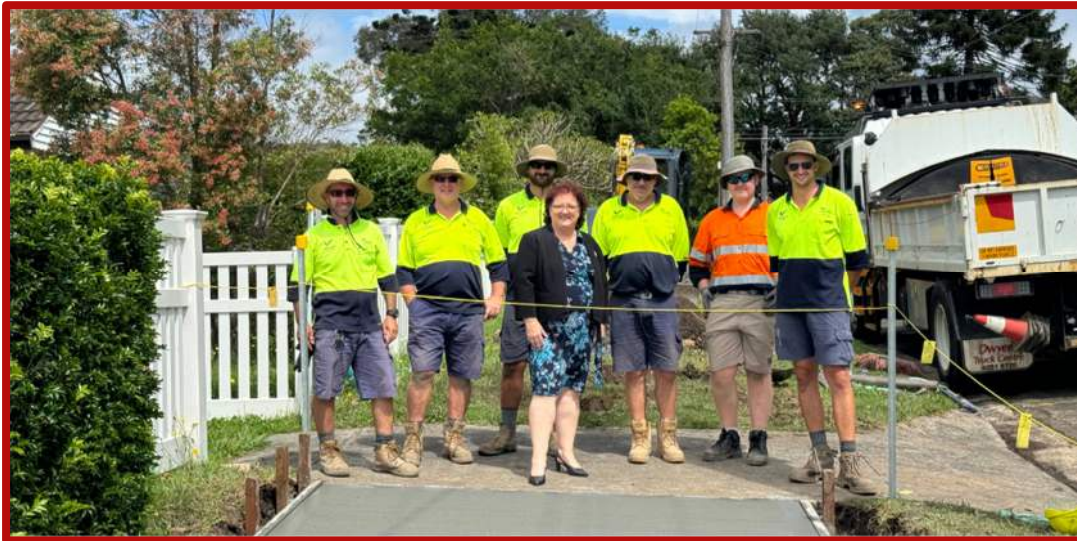
City of Wollongong Lord Mayor Councillor Tania Brown and Council staff at footpath works on Reserve Street, Wollongong.
