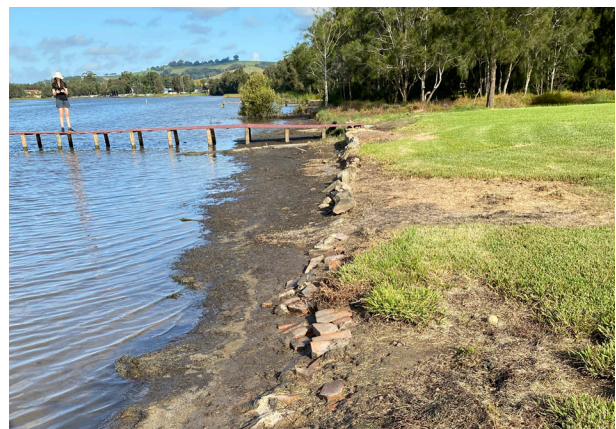
Run-down foreshore protection structures
