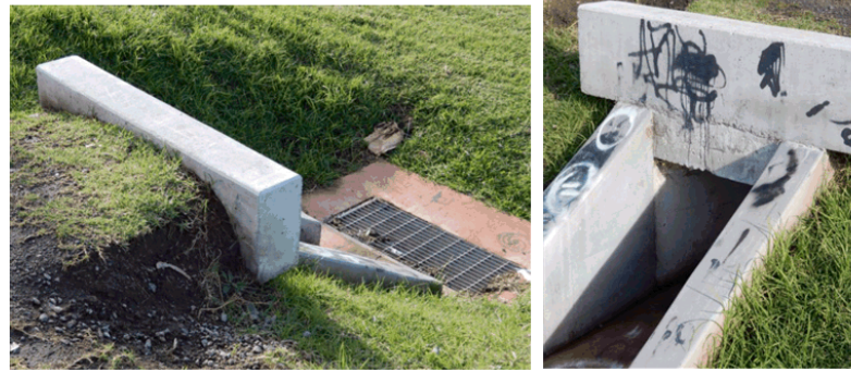
Drain covered in graffiti and creating a trip hazard.
