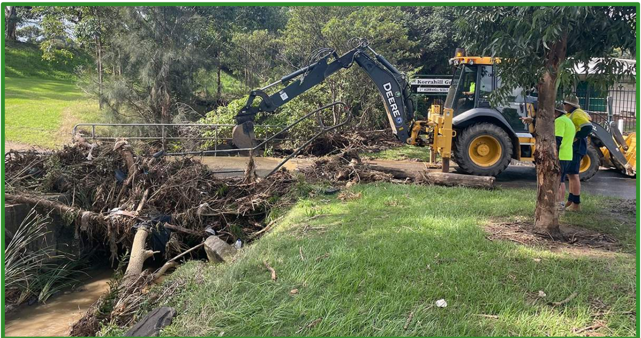
Council crews cleaning up debris at Russell Vale following the severe weather event on 6 April 2024.
