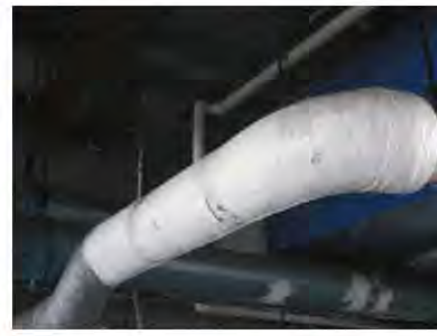
Figure 3: Friable Asbestos – Pipe Lagging
