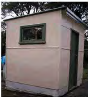
Figure 1: Bonded Asbestos (Fibro)
