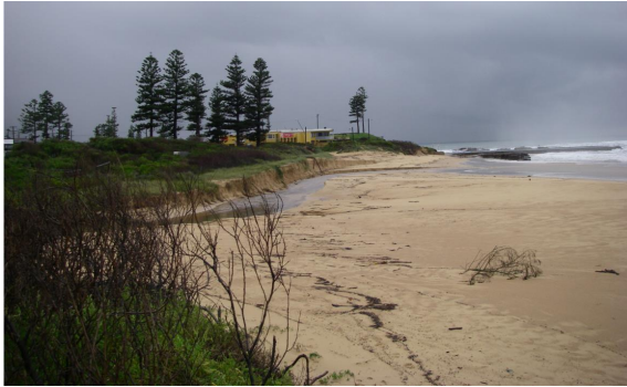
Plate 1 Breakout channel scour (WCC 28/6/2014)
