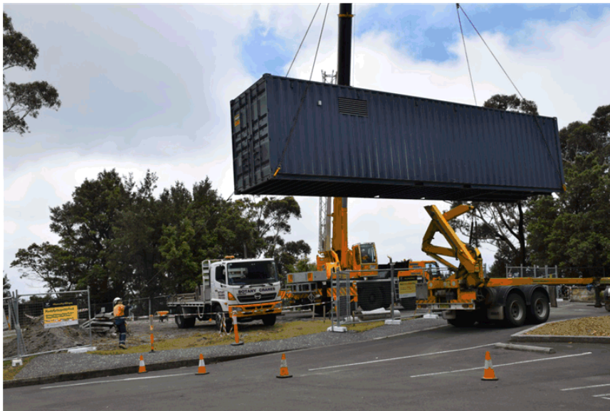
IMAGE: Installation of the Container Kiosk at Mt Keira. To improve the visual amenity of the container, an art work was also commissioned and delivered on the outside of the facility.
