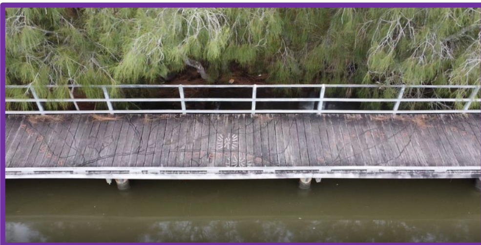
Hooka Point Berkely, work commenced on replacing the ageing timber deck of the jetty and footbridge as well as working with artists to repair and maintain as many of the existing artworks as possible.
