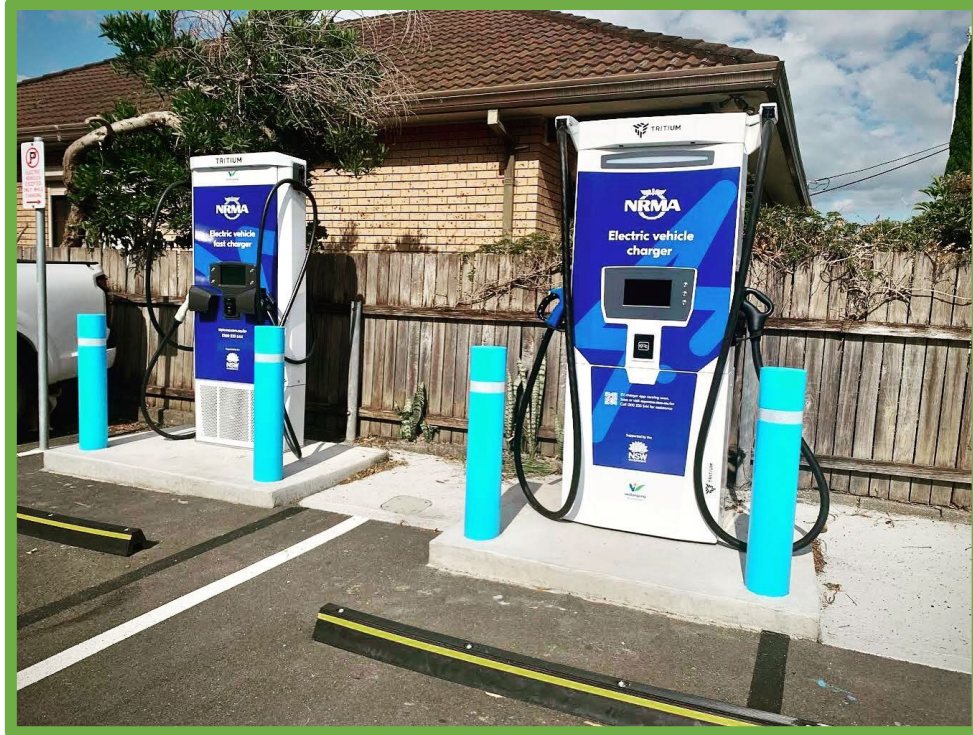
Installation new electric vehicle charging infrastructure at Stewart Street East Carpark, facilitated by the Electric Vehicle Charging Infrastructure on Public Land Council Policy.
