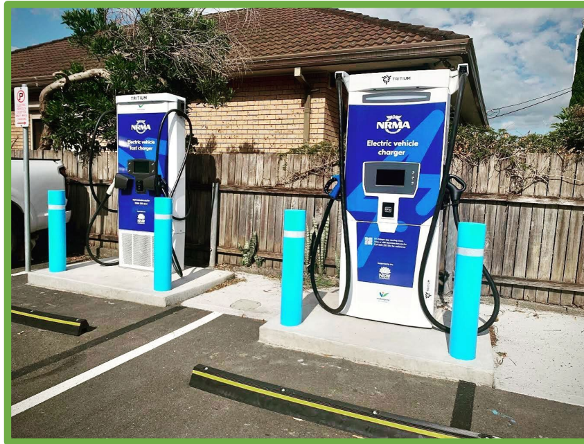
Installation new electric vehicle charging infrastructure at Stewart Street East Carpark, facilitated by the Electric Vehicle Charging Infrastructure on Public Land Council Policy.
