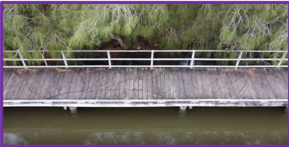
Hooka Point Berkely, work commenced on replacing the ageing timber deck of the jetty and footbridge as well as working with artists to repair and maintain as many of the existing artworks as possible.
